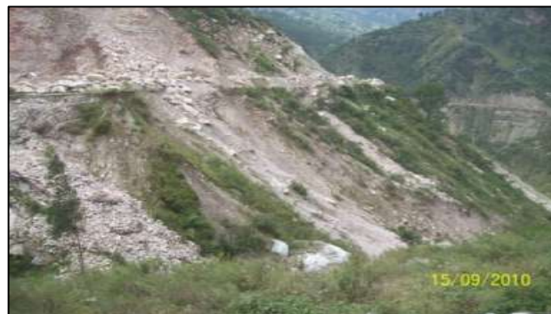
Plate 5.6 - Faulty Rock Cutting Resulting into Collapse of Slope
