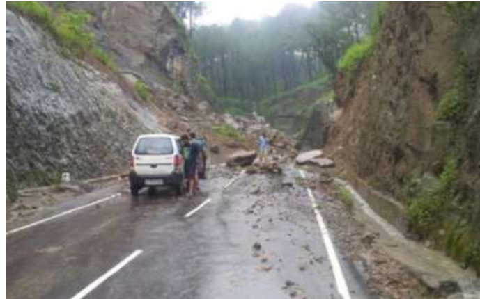
Plate 5.5 – Faulty Rock Cutting for Road Construction
