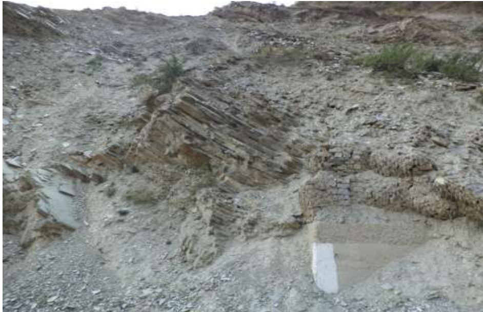
Plate 5.3 – Pandoh Landslide Blocking the Road
